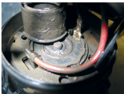
Corrosive exhaust gas condensate in the drive motor of a secondary-air pump
